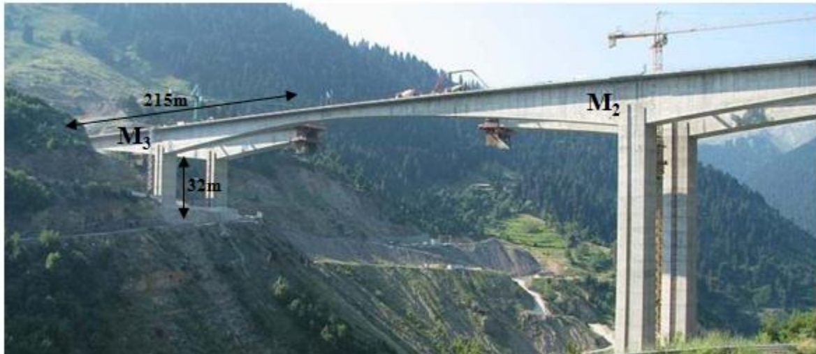
Figure 1: Metsovo bridge M_3 pier-deck segment prior (background) and after its connection with the M_2 pier-deck segment (foreground).
