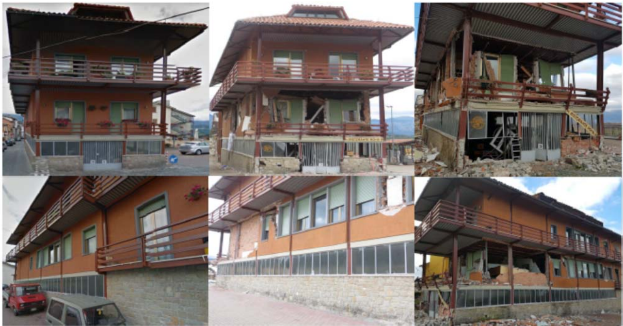
Figure 1. – Seismic response of the sample building: before the earthquakes (left), after the 24th August event (middle) and after the 30 th October 2016 (right).
