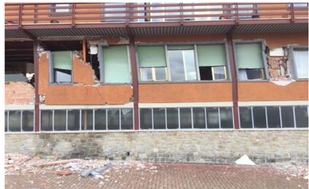
Figure 5. – Damage in the columns of the first floor of the building
