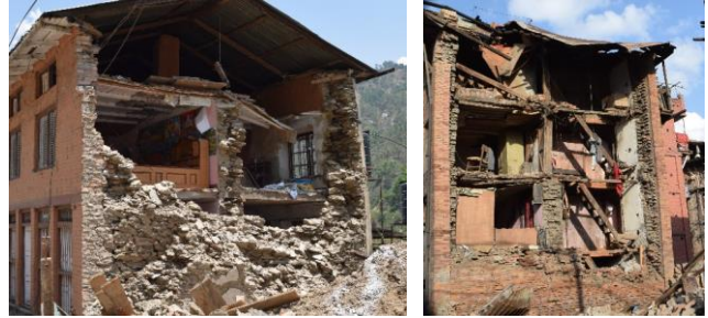
Figure 1: Out-of-plane damage of Nepalese URM buildings (credits: Rama Mohan Pokhrel).
