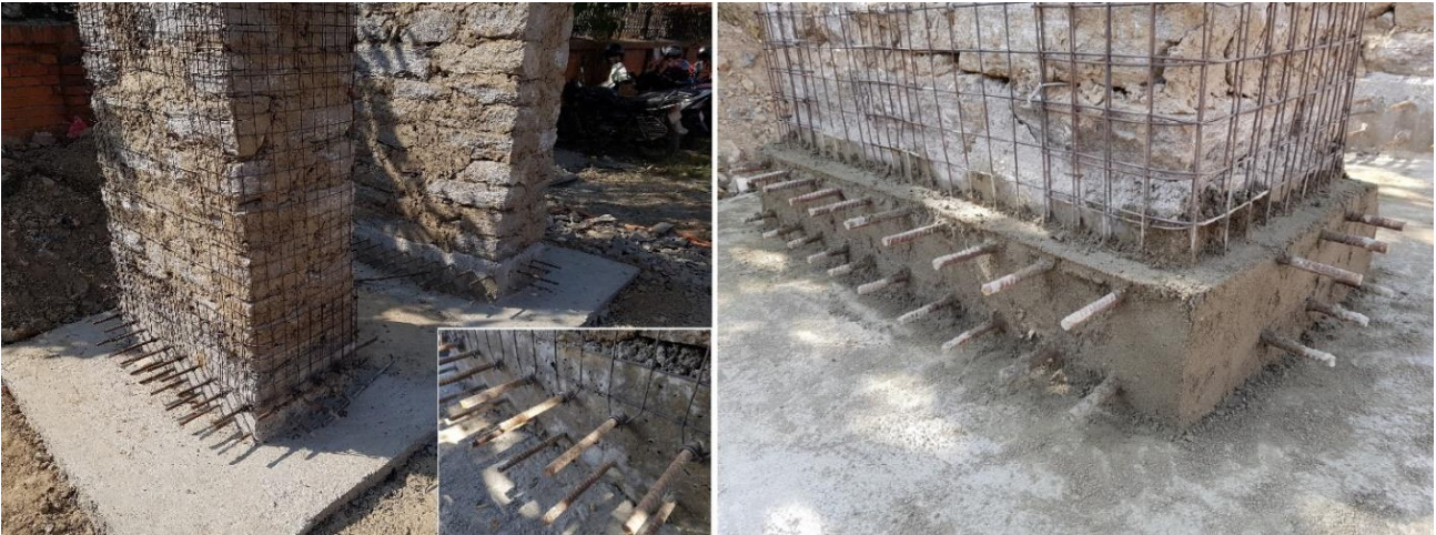
Figure 4 Wire mesh tied and welded to the rebar of the pedestal (left); Connections covered with 50mm of 1:6 plaster (right)
