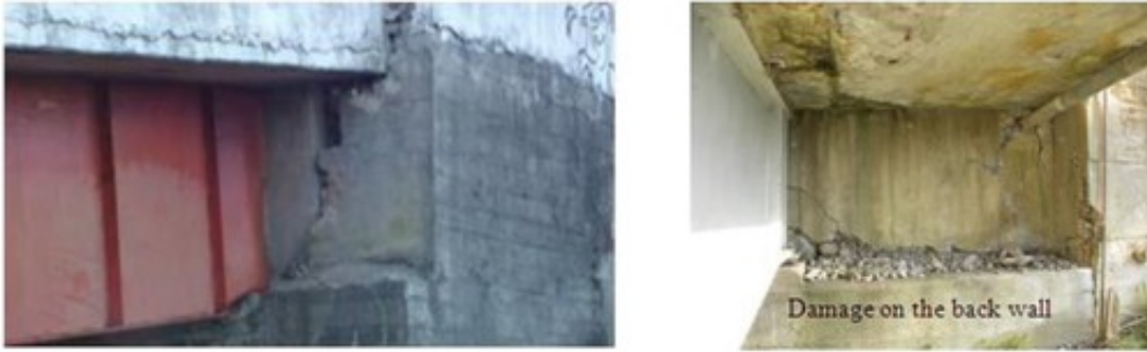
Figure 2. Examples of backwall damage: (left) punching of the Tubul bridge deck into the backwall, and (right) damage at the base of the abutment backwall of the El Bar bridge. After Zheng et al. (2021).
