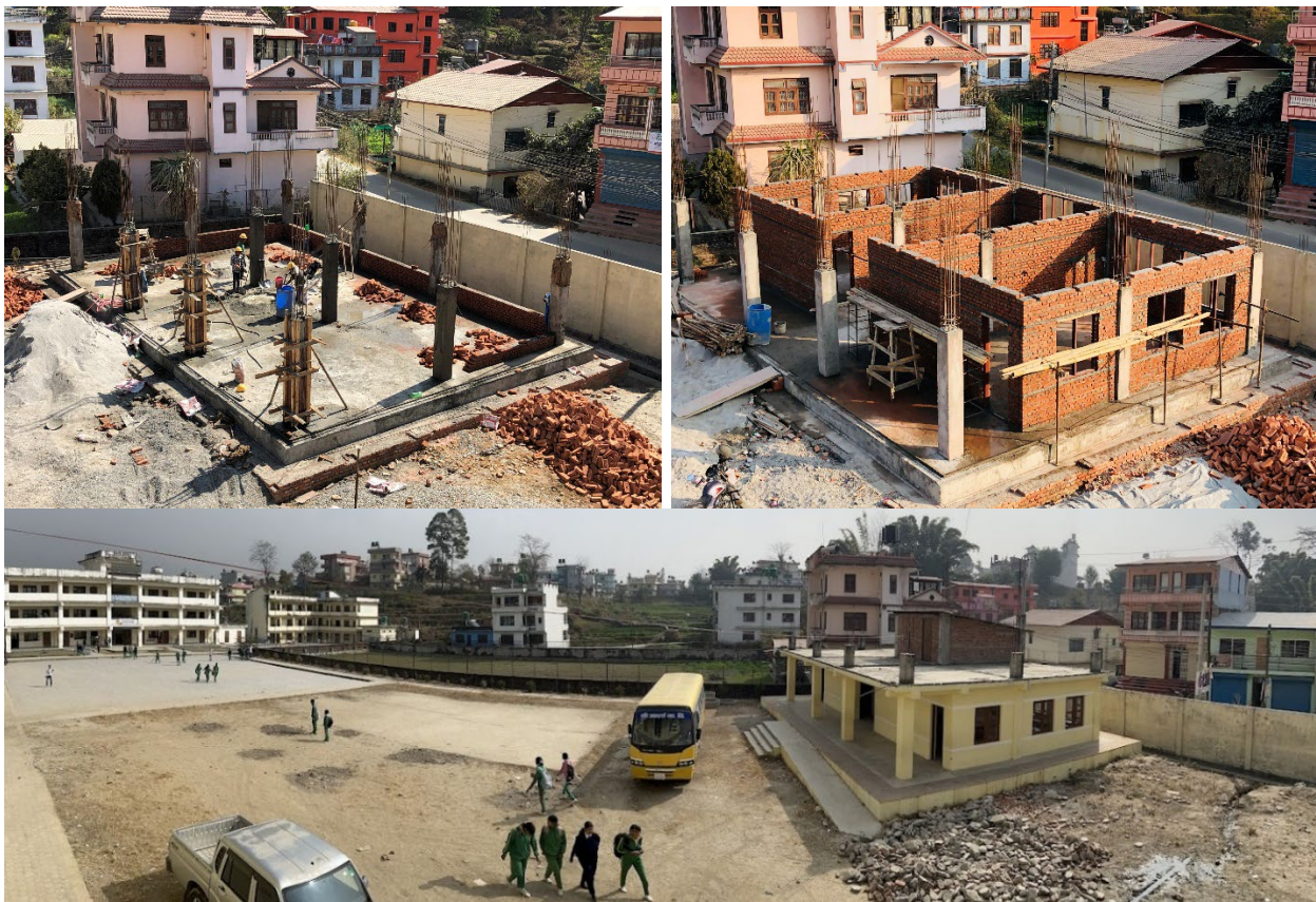
Figure 4.4 Finalization of the superstructure construction (top) and delivery of the operational school (bottom).
