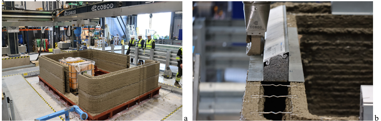
Fig 5. (a) first printed layers of the housing unit; (b) Use of lintels in the 3D-printed walls of the housing unit at SOFSI Lab.
