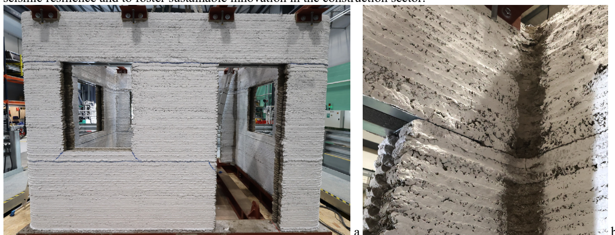
Fig. 6. (a) Cracking mechanism observed in the 3D-printed housing unit during the final seismic test; (b) an interior view of the crack in the dry joint at the top of the opening.
